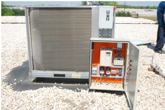
Installation of the Energy Savings Equipment onto a standard (Unmodified) "Carrier" HVAC System
